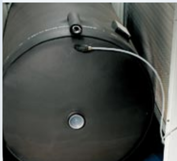
Large buffer tank
